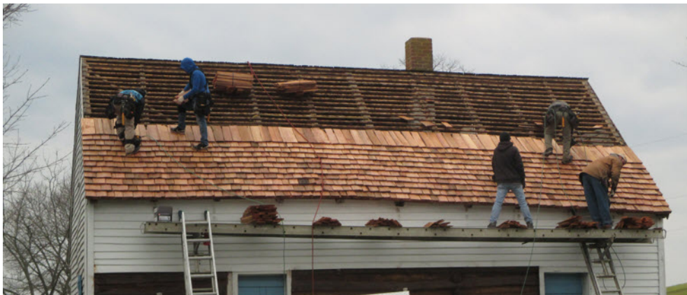
The new roof for the Log Meeting House will look much like this one, seen here as it was installed on the Evans House last year - being made of wood shingles and laid as it would have been in 1764.
